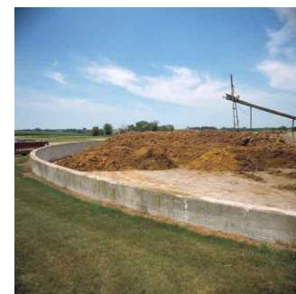
Photograph of a manure storage facility. Photo: Ontario agriculture photo library
